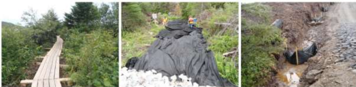
Figure 11. Some mitigation strategies for access roads: wooden boardwalk to minimize impact of access to sensitive areas (left), geotextile layer (centre), silt fence check dam (right).
